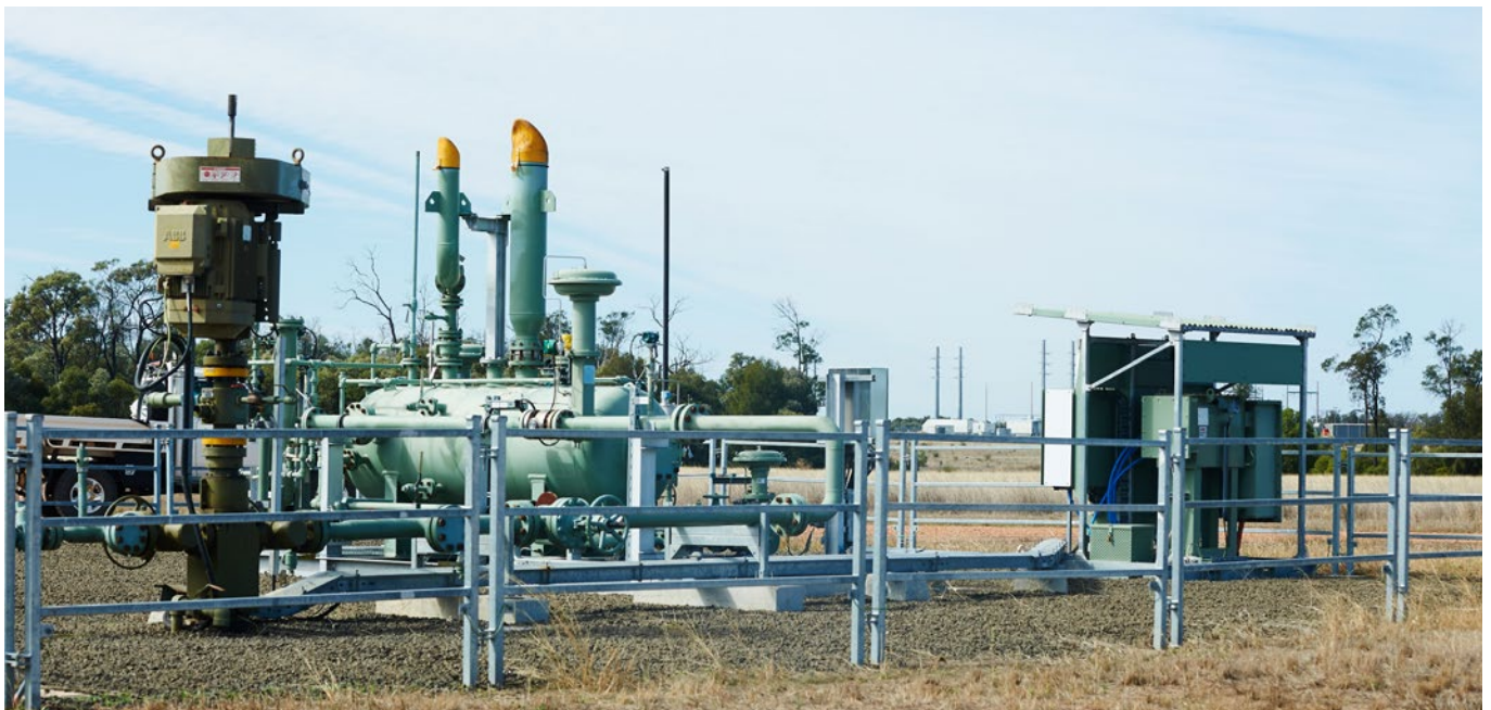
A coal seam gas well head.
