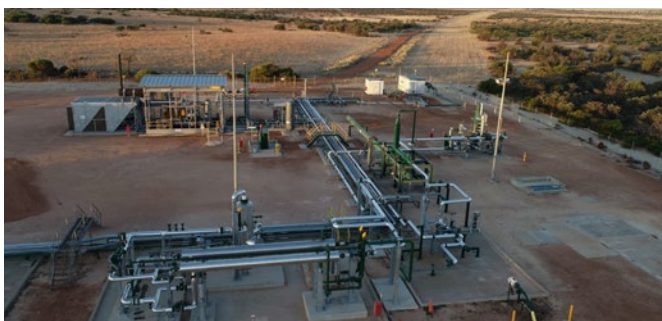
Onshore gas facility in the northern Perth Basin.
