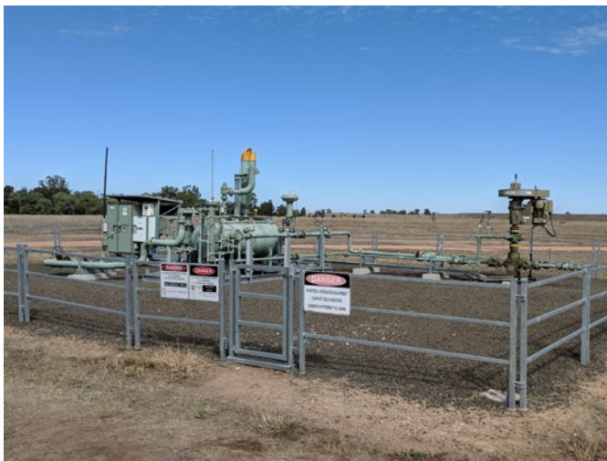
A CSG well head in the Surat Basin, Queensland.
