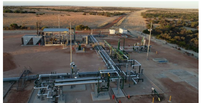
Waitsia gas field infrastructure. Banner image: Mid West region landscape.
