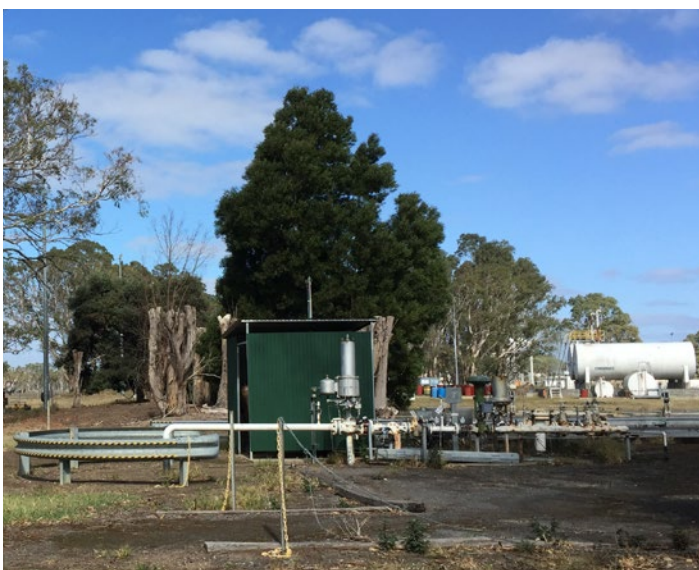
Conventional gas well head infrastructure near Penola. This project will review the role of gas in future scenarios.
