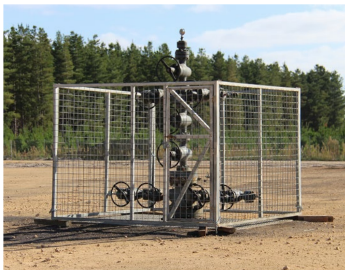
The Hasselgrove 3 conventional natural gas exploration well head near Penola.
