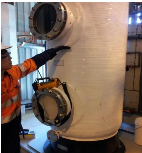
Figure 3: Activated alumina vessel in SG WTF – August 2013.
