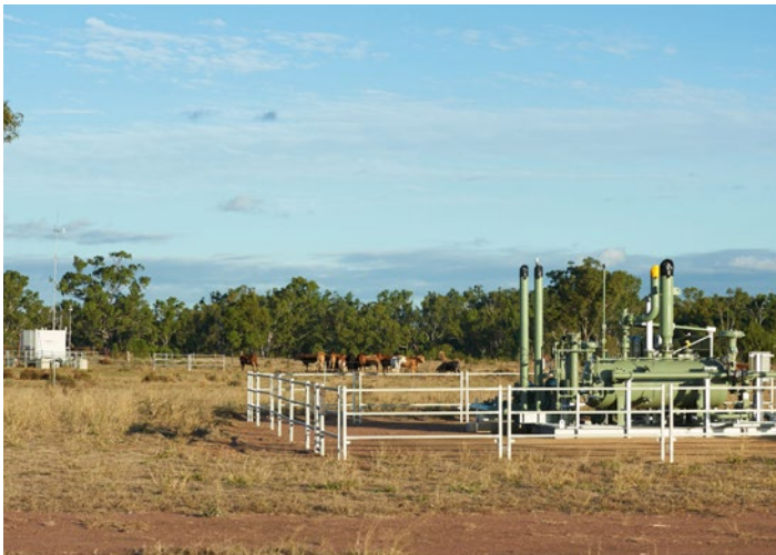
Coal seam gas well and an air monitoring station in the background.
